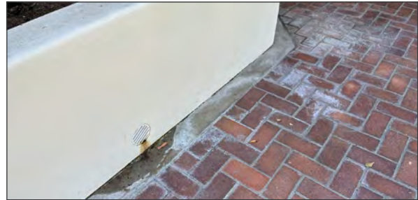
Heavy water stains and efflorescence at brick paving (ARG, 2023).
