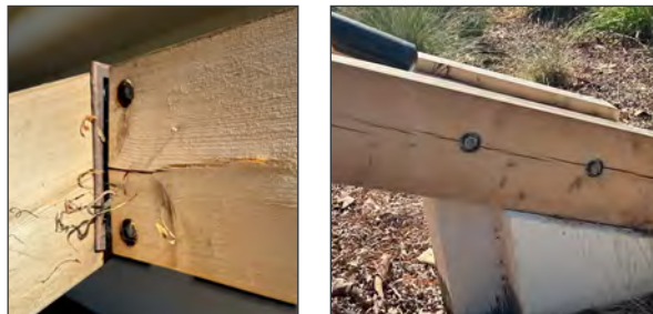
Details of splitting at wood trellises (ARG, 2023).
