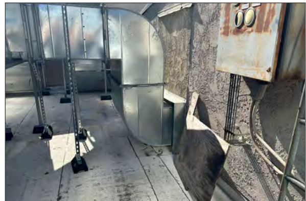
Air handling unit at roof (ARG, 2023).
