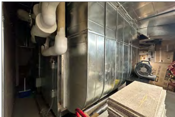
Air handling unit in basement (ARG, 2023).
