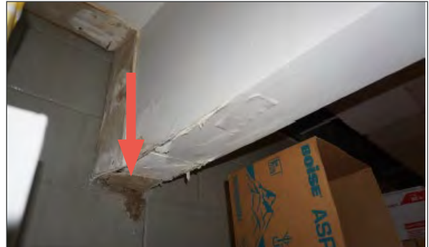
Moisture damage on gypsum wall boards abutting the CMU foundation wall, indicated by red arrow (WJE, 2023).
