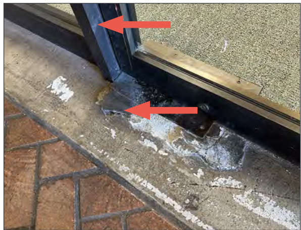
Detail of concrete damage, poor previous patches, and oxidation of aluminum storefronts, indicated by red arrows (ARG, 2023).
