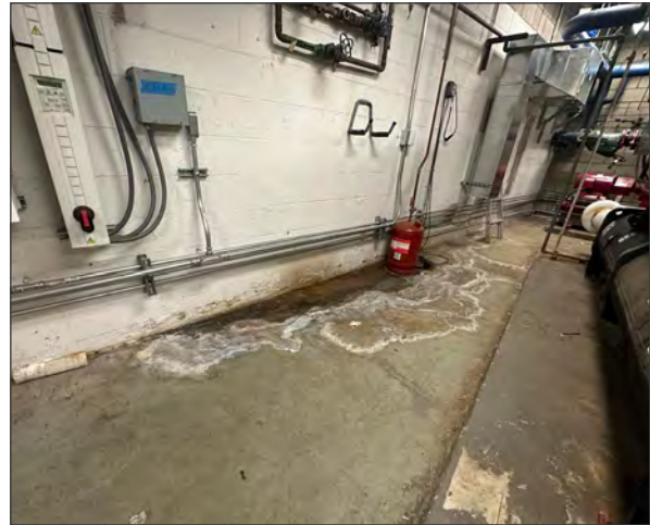
Basement chiller room (ARG, 2023).
