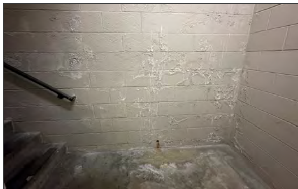
Peeling paint and water stains at CMU basement wall (ARG, 2023).
