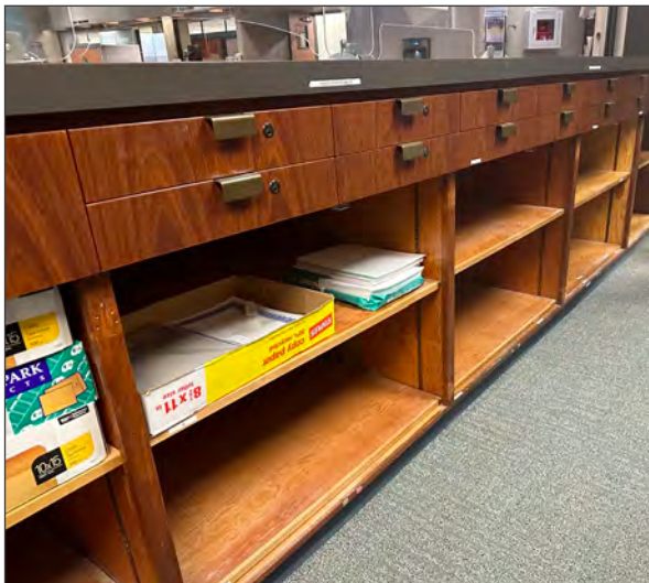
Missing cabinet doors at counters (ARG, 2023).
