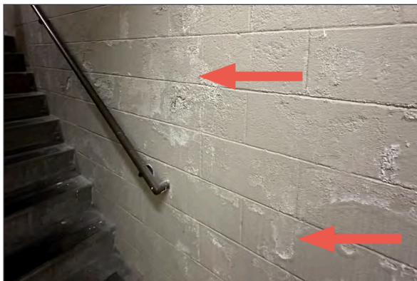
Peeling paint and efflorescence at basement CMU north exit stairwell wall, indicated by red arrows (ARG, 2023).
