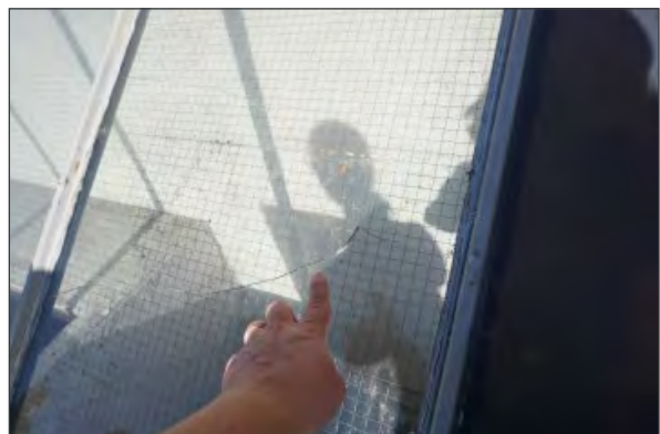
Close-up of cracked skylight glass (WJE, 2023).
