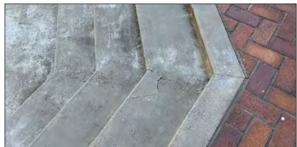
Cracking and efflorescence at concrete steps (ARG, 2023).
