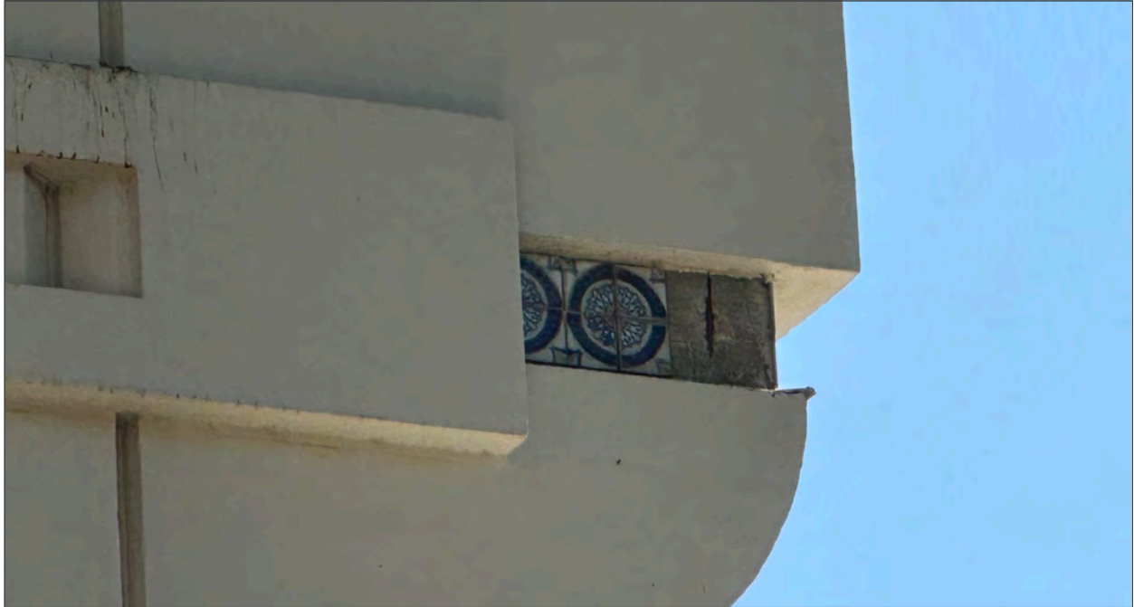
Missing tile at overhang above south entrance (ARG, 2023).
