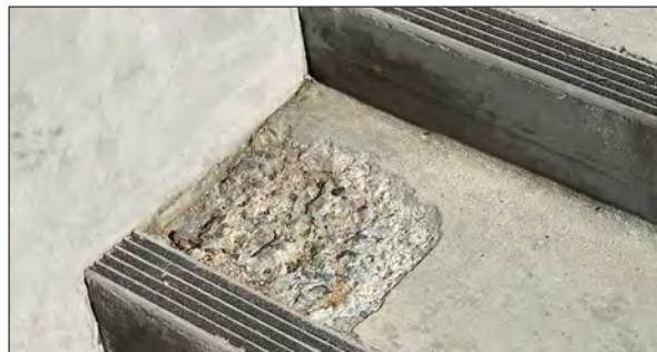
Detail of concrete spall at plaza steps (ARG, 2023).
