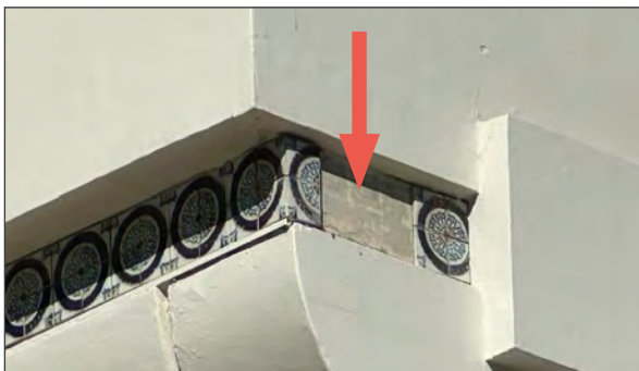
Detail of missing tile above southwest wing (ARG, 2023).
