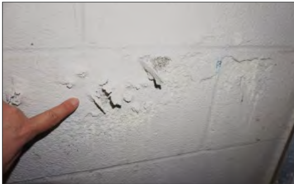
Blistering and debonded paint on CMU foundation walls (WJE, 2023).
