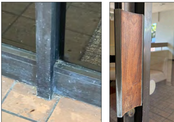
Oxidation at aluminum storefront (left) and irregular surface wear at cedar door pull (ARG, 2023).
