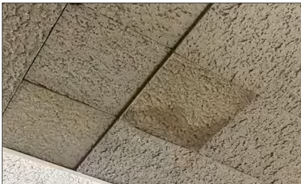
Detail of stained acoustical tiles (ARG, 2023).
