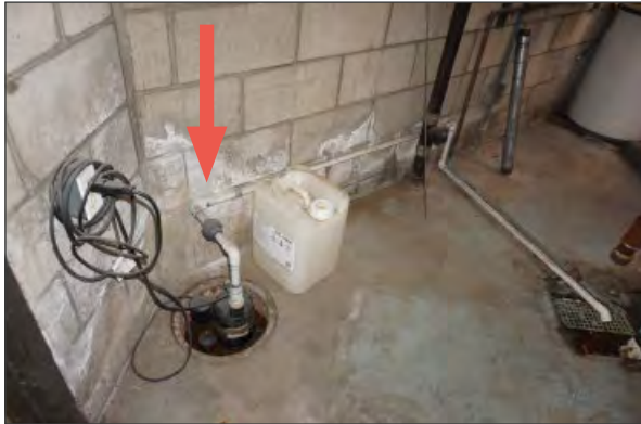
Typical efflorescence on CMU foundation walls, indicated by red arrow (WJE, 2023).
