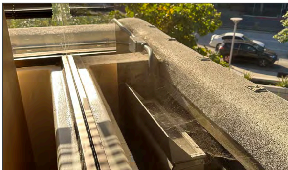
Exterior planter at the second floor that wraps around to the southwest wing, east and west façades (ARG, 2023).
