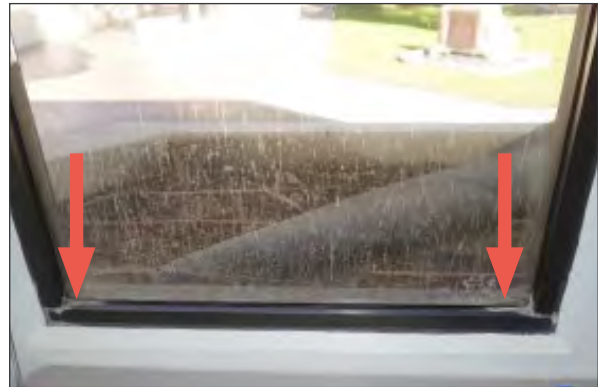
Interior view of water staining at window corners (WJE, 2023).
