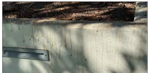
Water stains at concrete planter walls (ARG, 2023).
