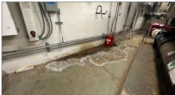
Basement chiller room (ARG, 2023).
