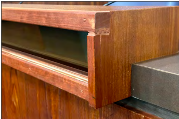
Damage at council desk millwork (ARG, 2023).
