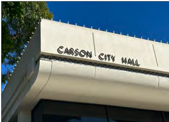
View of tile along overhang at the southwest wing, south façade (ARG, 2023).
