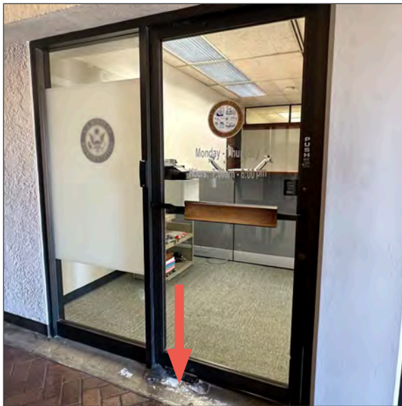
Damaged concrete threshold at corridor office doors, indicated by red arrow (ARG, 2023).
