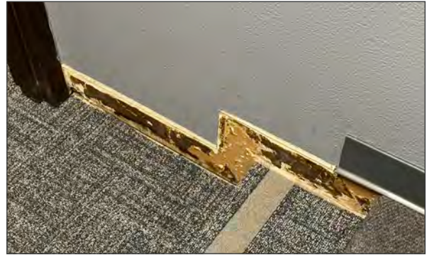
Detail of missing rubber base trim along the west interior wall (ARG, 2023).
