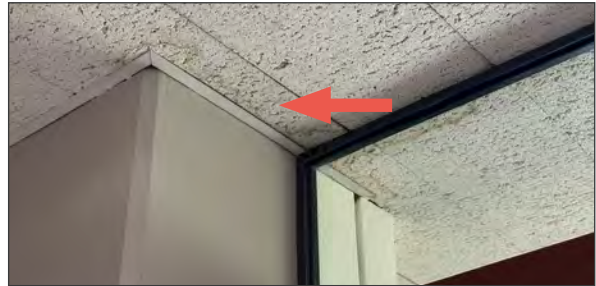
Localized areas of water stains at acoustical tiles, indicated by red arrow (ARG, 2023).
