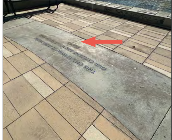
Crack at engraved concrete paving, indicated by red arrow (ARG, 2023).
