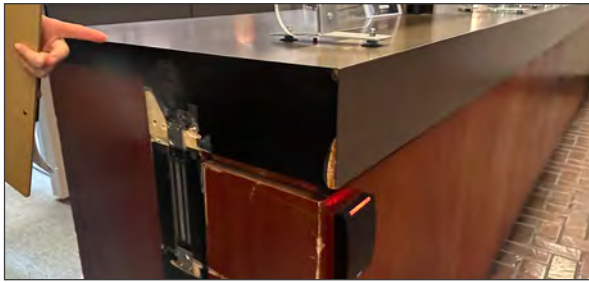
Missing gate/door at counter and damaged laminate countertop (ARG, 2023).
