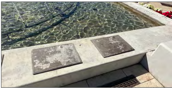
Deteriorated plaques at plaza fountain (ARG, 2023).
