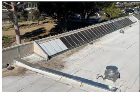
View of skylights painted/covered with plastic sheet (WJE, 2023).
