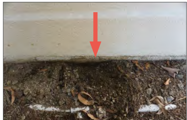
Exposed wall condition at planters with exposed mesh reinforcement at new plaster finish indicated by red arrow (WJE, 2023).
