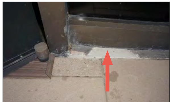
View of storefront system sill from the exterior. Exposed concrete floor slab and evidence of repair indicated by red arrow (WJE, 2023).
