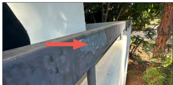
Peeling paint at balcony railing at the east end of the east wing, indicated by red arrow (ARG, 2023).
