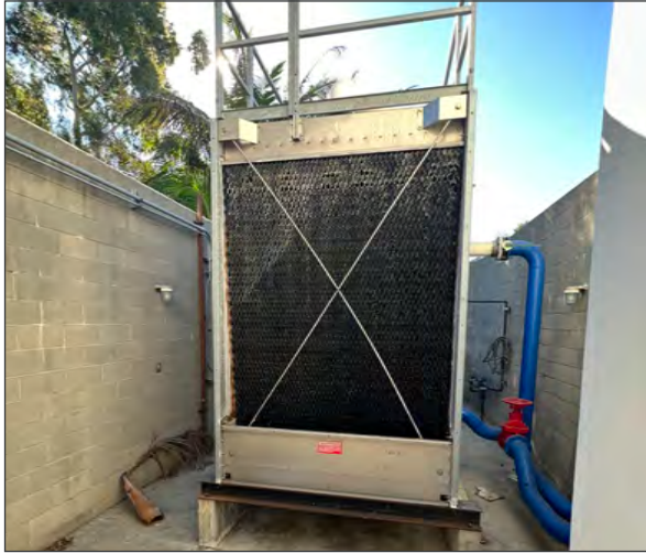
Cooling tower at roof (ARG, 2023).
