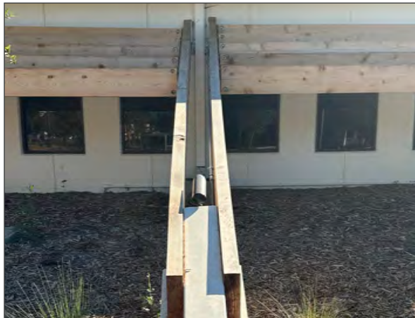
Checking and splits at wood trellis framing (ARG, 2023).
