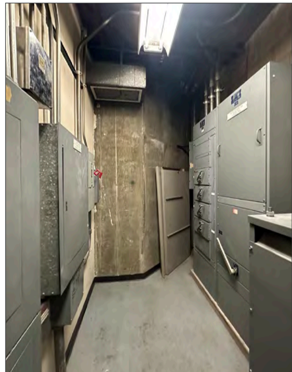
Basement electrical substation (ARG, 2023).
