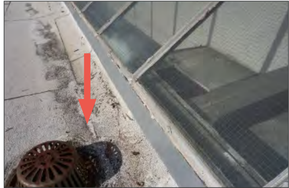
View of debris and granule accumulation at roof low spots , indicated by red arrow (WJE, 2023).
