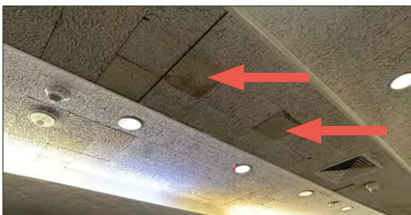
Stained and damaged ceiling tiles, as indicated by red arrows (ARG, 2023).
