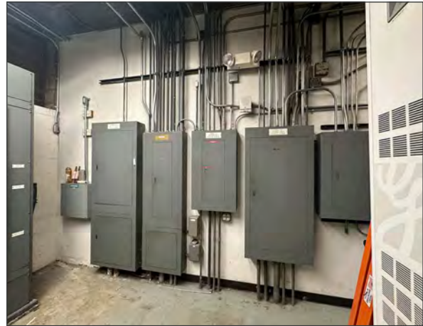
Basement main electrical room (ARG, 2023).
