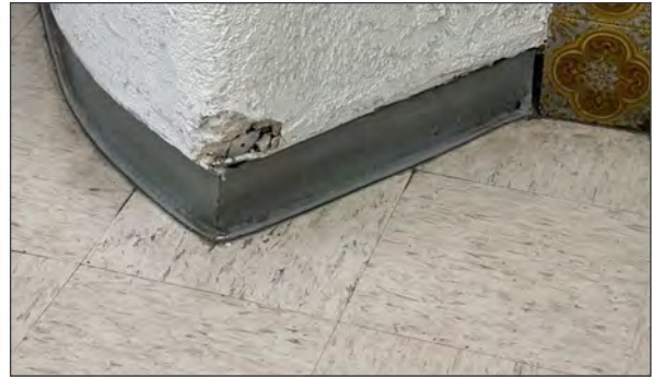
Spalled plaster next to the basement elevator (ARG, 2023).
