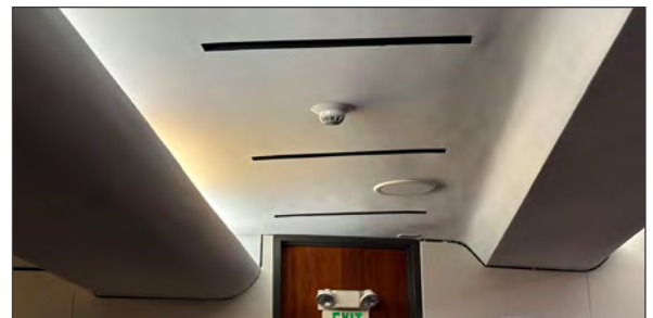
Plaster ceiling with soffit lighting and plaster walls in the council chambers (ARG, 2023).
