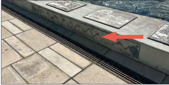
Missing tiles at plaza fountain, indicated by red arrow (ARG, 2023).
