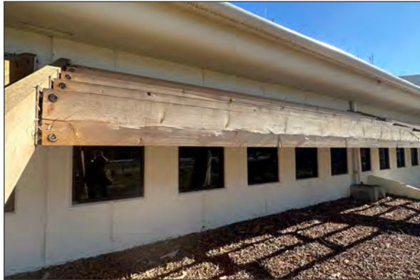
Checking and splits at wood trellis framing (ARG, 2023).
