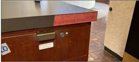
Missing plastic laminate at countertop (ARG, 2023).
