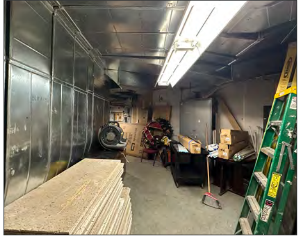
Basement air handling unit (ARG, 2023).
