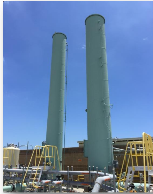
Landfill Gas Collection System
