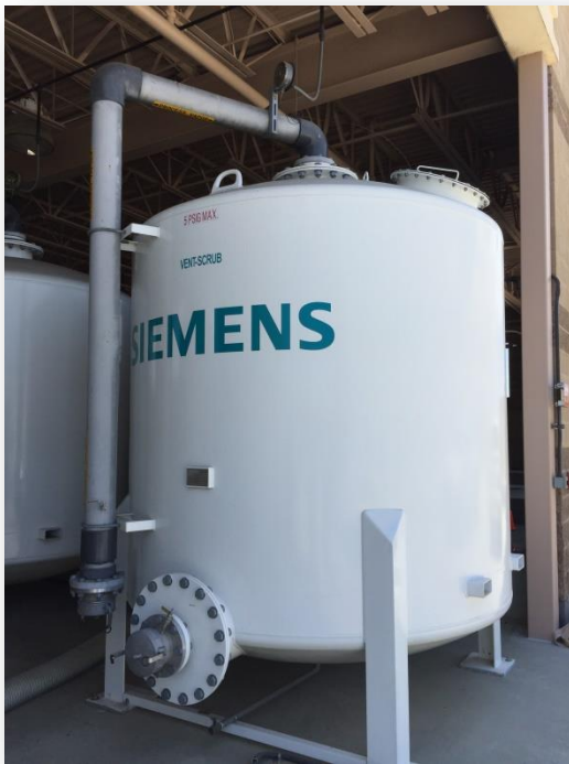
Groundwater Extraction System
