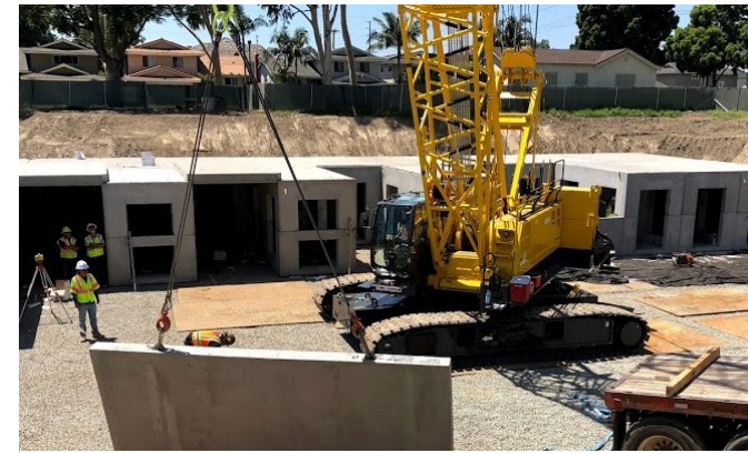
Craftwater Engineers led the analysis and design of the award-winning Caruthers Park SW Capture Project.
