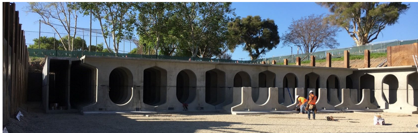
Figure 5-2. Craftwater Engineers led the implementation of Lakewood Bolivar Park regional stormwater capture project under an accelerated design and construction schedule.
